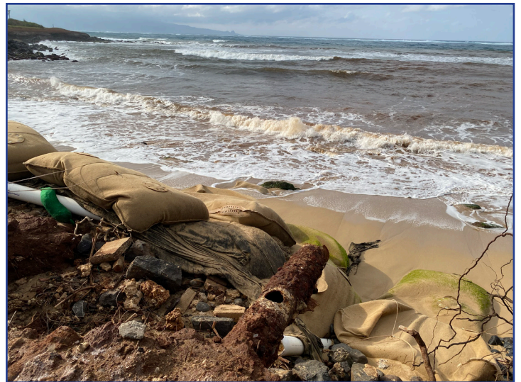
Many bags of the shoreline structure have been displaced during the enormous swells in December and January and continues to weaken the bank.
