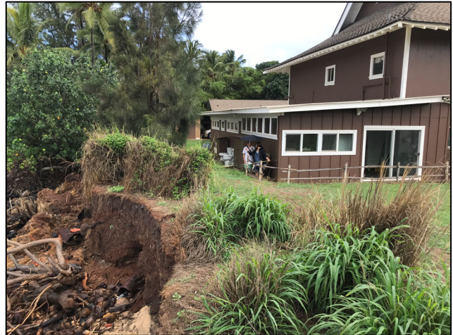
Figure 1: Photograph taken in January 2020, showing the erosion escarpment in proximity to the temple. At the time, the erosion escarpment was approximately 18 feet from the structure. Today it is much closer.
